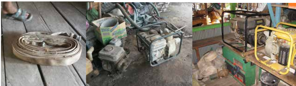
This fire fighting equipment has mostly never been used (C Kalimantan)
