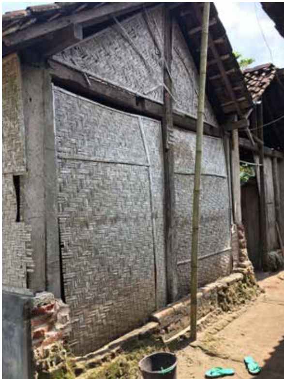
A 'gedek' house, built in some communities after the earthquake with the help of outside aid. These were generally meant to offer family's shelter in the months after the earthquake until they were able to fully rebuild their homes. Although simple, most people said they liked the gedek because that they 'can't hurt you' if there is another earthquake. Those that are still standing and/or haven't replaced in communities like Bantul hill and Bantul market are often being used for storage.
