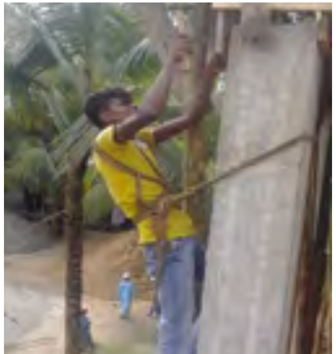
Rod binding worker with a self made belt hanging from the wall as he worked
