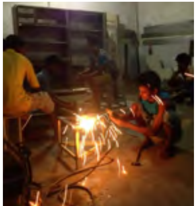
Steel worker with no protective goggles or equipment while welding.
