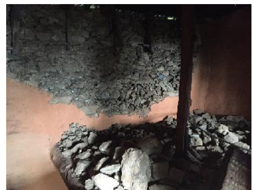
Wall that collapsed in an aftershock in Central Gorkha
